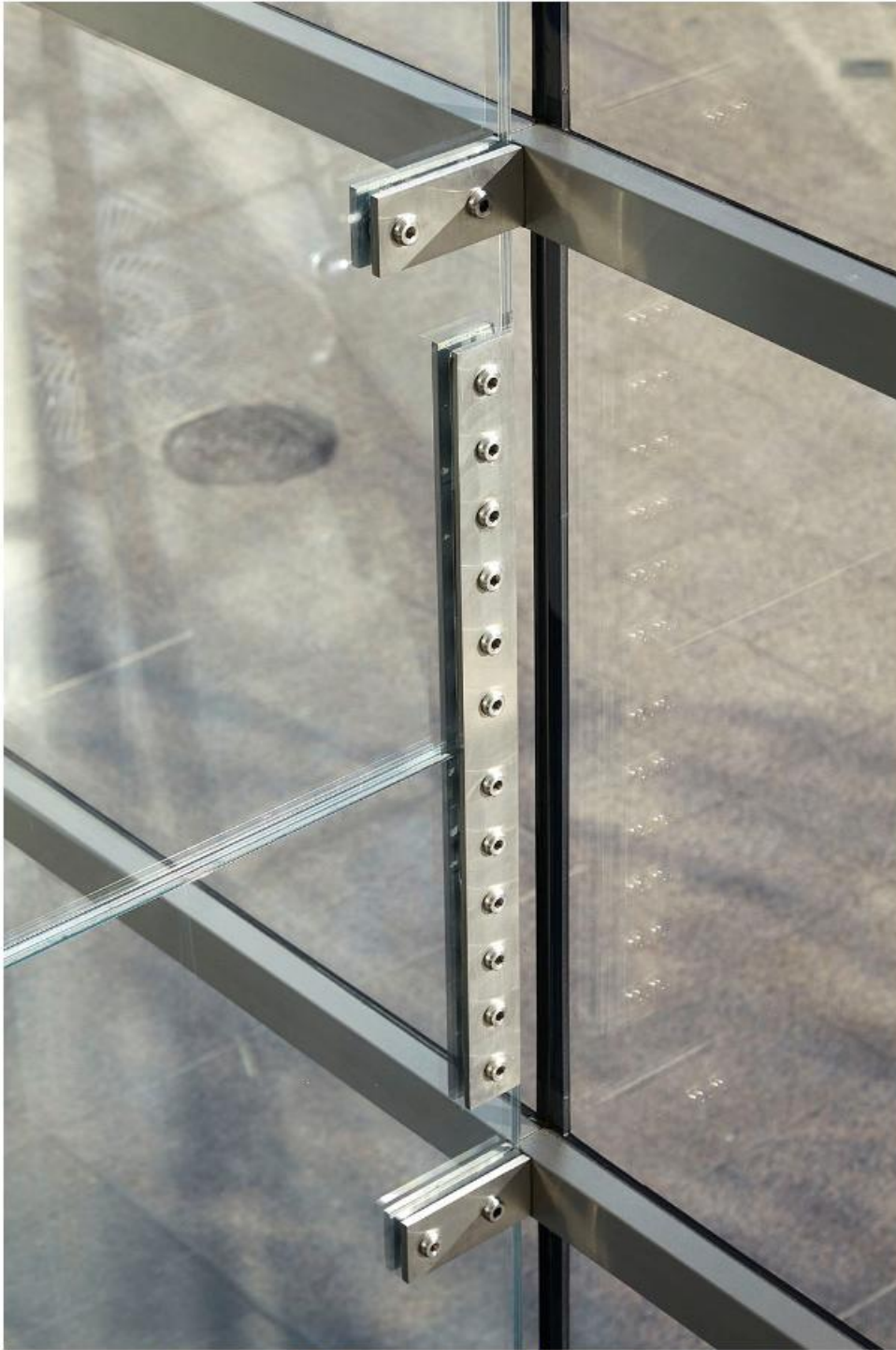
The 7m long glass fins bear the load of the all-glass façade. The connection parts are kept unobtrusive so that the transparency of the building envelope is hardly affected. (Photo: Greg West Photography)
